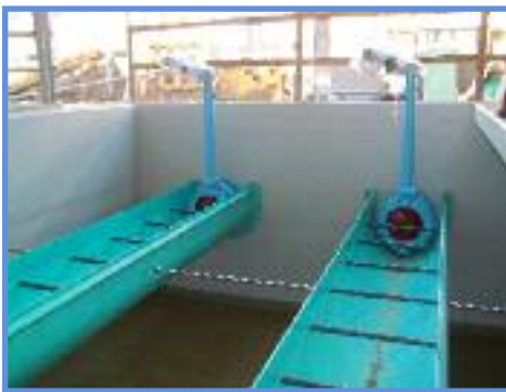
New conventional filter at Middle Fork Water Treatment Plant.
