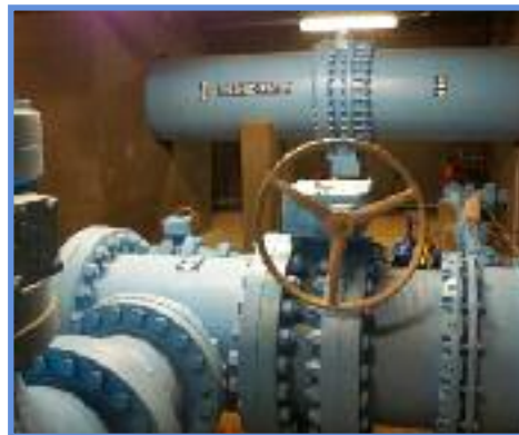
Finished water piping at Middle Fork Water Treatment Plant.
